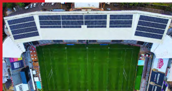
Durban, South Africa – 398 kWp rooftop solar installation under a PPA model.
