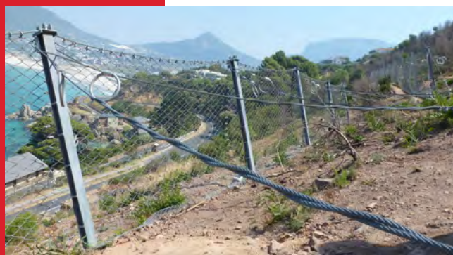
Chapmans Peak: shallow landslide barrier
